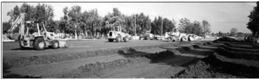
The base is the most important phase. It requires a precise grading strategy, the right material and good supervision
