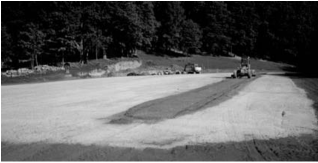
A grader is highly recommended to properly level the different layers of footing.
